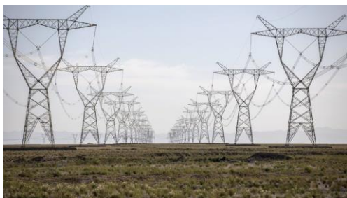
Figure 52. The 1,100-kV direct-current Changji-to-Guquan project stretches 3,293 km (2,046 miles). It is currently the world biggest UH voltage direct current power line. Image credit: Qilai Shen, Bloomberg
